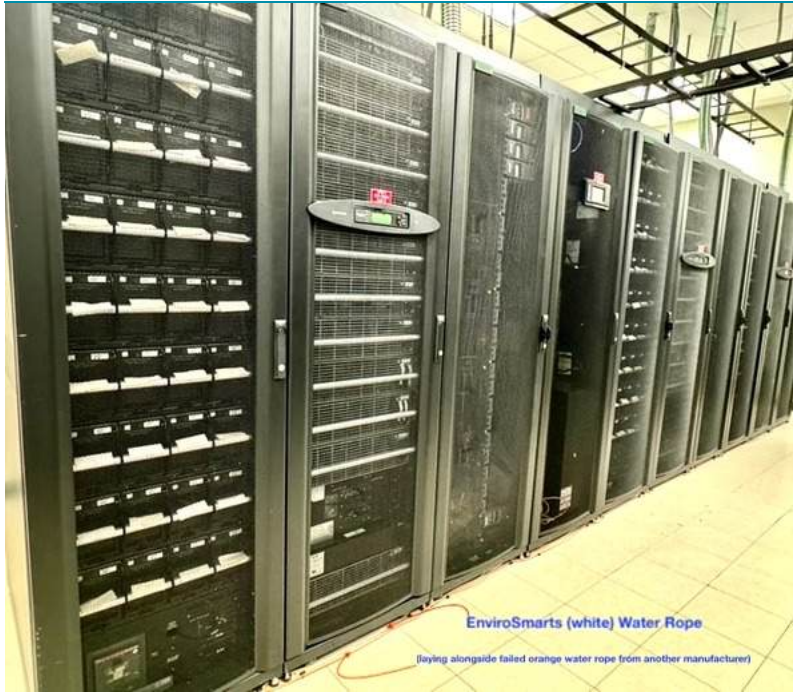
EnviroSmarts WLD sensor (with white water rope) deployed at CBOE Kansas City Backup Server Farm
